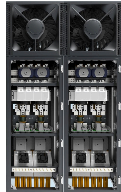
REAR — INNER DOORS OPEN ISOLATORS, FUSING, CONTACTORS, DC BUSBAR
